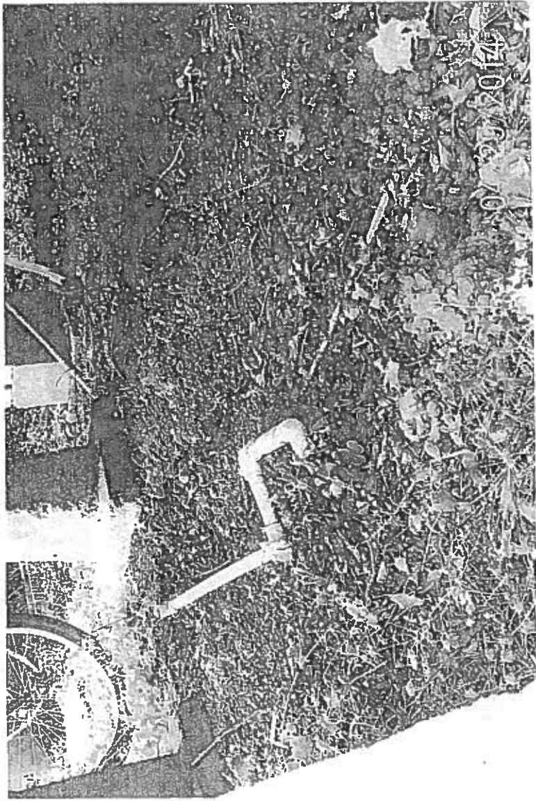
The receiver airline is broken.
