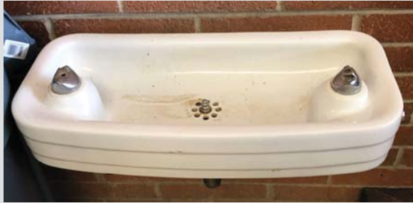
DF08 – BUBBLER IN ASSEMBLY ROOM NEAR CAFETERIA ENTRANCE
