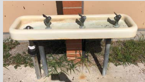
DF09 – BUBBLER OUTSIDE IN PLAYGROUND FOR PREK HARD DISCONNECTED
