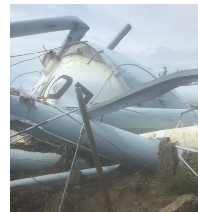
Houma Area WS – Lower Terrebonne (Dulac) Elev Tower collapse
