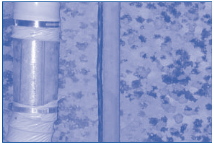
Photo above: mold growing on backside of wallboard.
