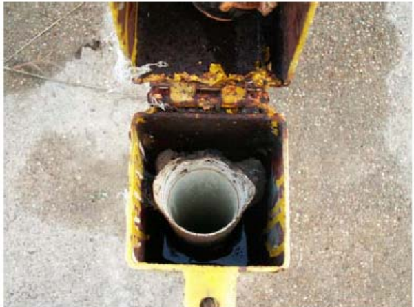
File Name: GSV_photo8.JPG Date/Time Taken: 01 Oct 2005 1733 Description: Warped top of riser pipe, well D-3R. N29°57'26.2"; W92°11'13.1"
