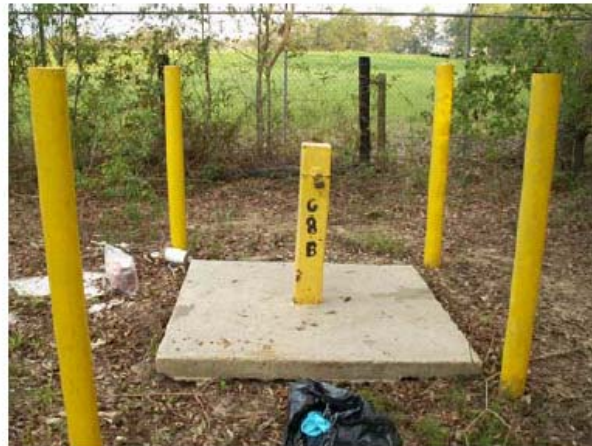
File Name: GSV_photo10_WellPad_G-8D-3.JPG Date/Time Taken: 01 Oct 2005 1730 Description: Well G-8B (location for sample GCV002). N29°57'26.8"; W92°11'14.4"
