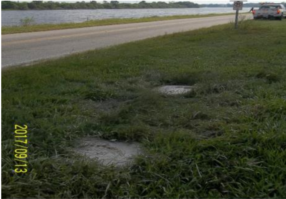
Looking northeast across two flush mount monitoring wells. The sampled well MW-7 is the furthest well (near the center of the picture).
