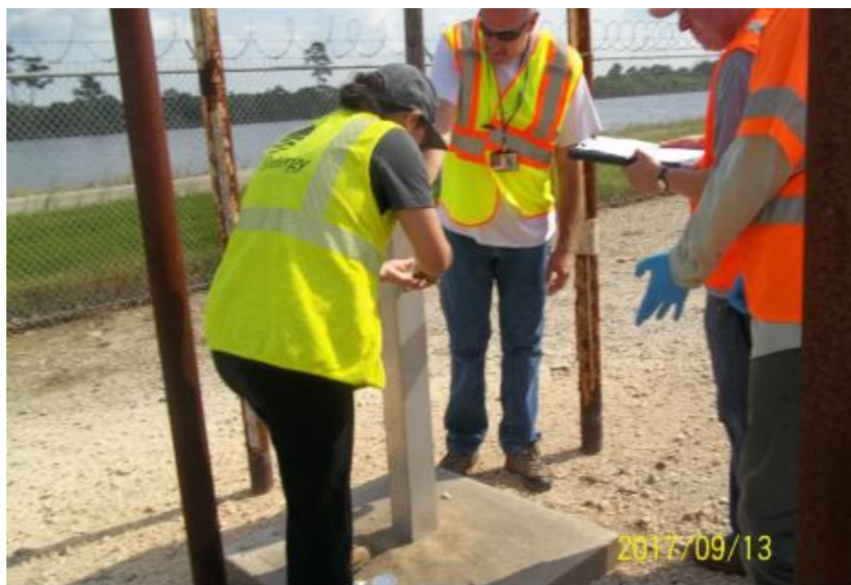
Opening monitoring well 1 (MW-1), looking northeast toward road and river; this is the well where sample GSU-GW-002 was collected. Date/Time: 09/13/2017 10:09 a.m.
